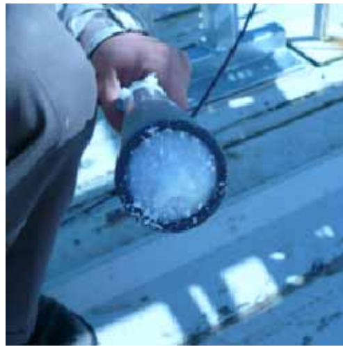
Ice build-up inside ASD pipe (ice plug)
