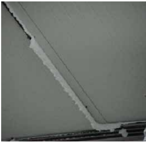
Ice build-up on ASD sampling holes
